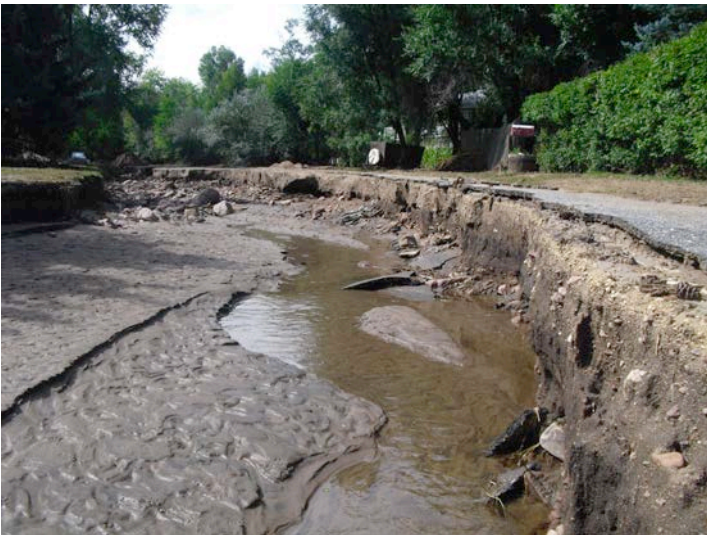
Fourmile Canyon Creek overflow path along Topaz Drive. Source: UDFCD
