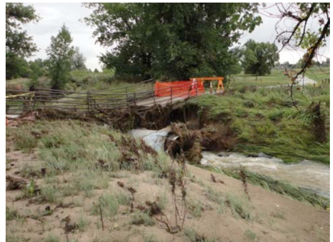
Post Flood Trail Damage
