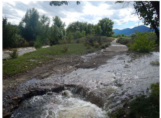
South Boulder Creek bike path washed out near U.S. Highway 36. Source: CH2M HILL
