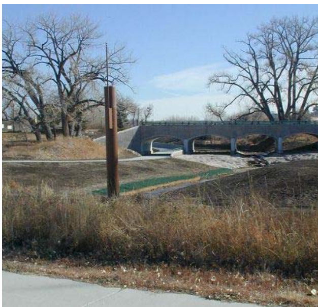
The new ALERT gage on Sulphur Gulch in Parker
