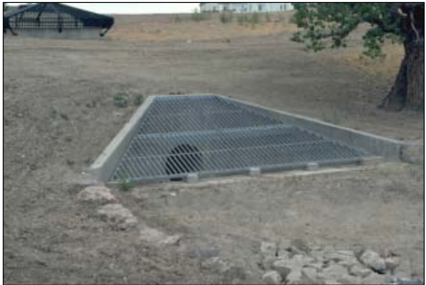
An example of a trash rack (from the USDCM)
