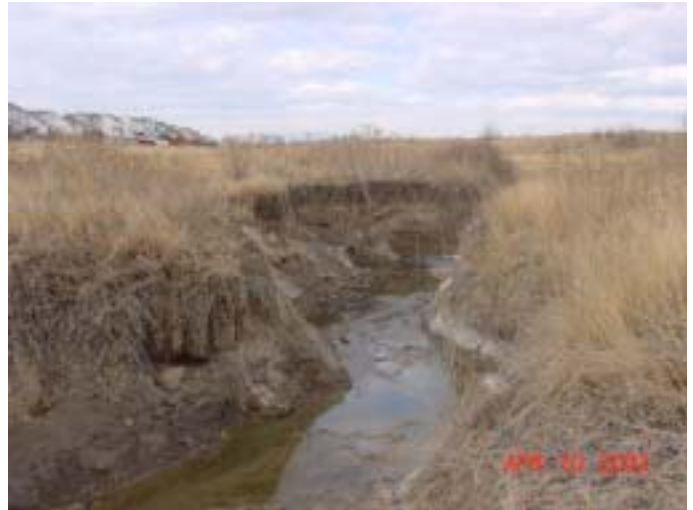
Brantner Gulch looking upstream (West) approximately one-half mile downstream of Holly Street
