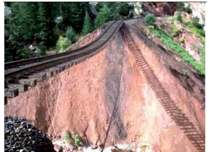
Bull Gulch post-flood railed railroad embankment (looking north). Source: Michael Baker International
